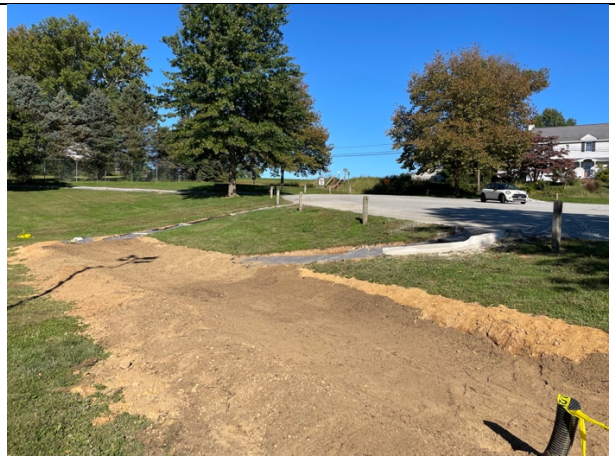
Construction Day 5&6 – Emergency drain, bioretention mix, rock for inlets, and mulch added.
