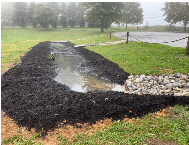
1” rain event prior to planting (water had to be pumped out so the planting could occur)
